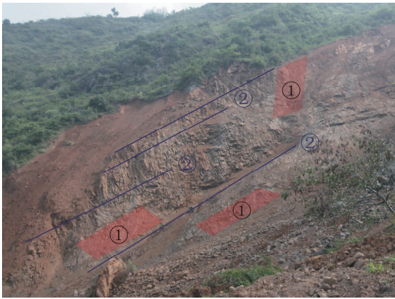
圖7 滑源區斜坡岩體的兩組主要結構面 Fig.7 Two main discontinuities of the slope rock mass in source area
